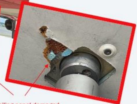
Ceiling panel damaged
